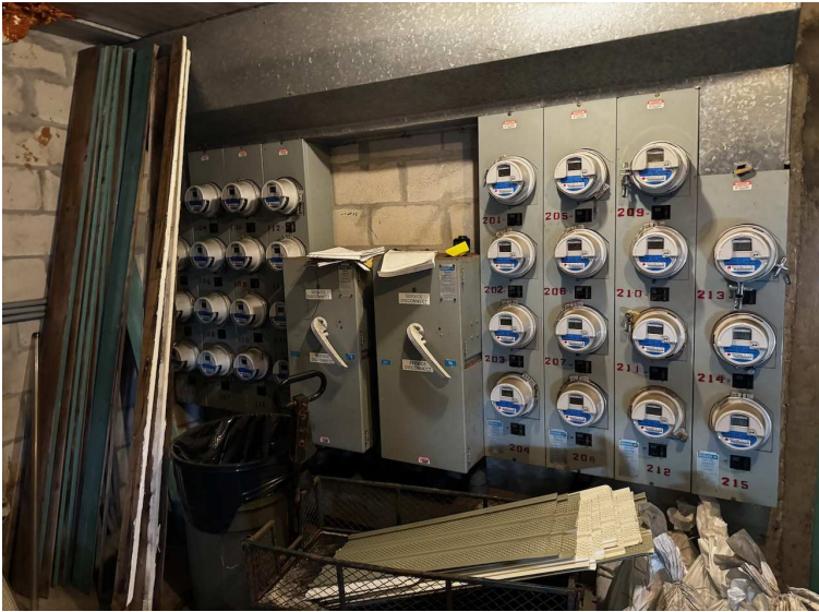
Panels and meter sockets.
